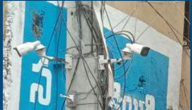
Installation of CCTV cameras at Jubilee Hills, Madhura nagar, Film Nagar & Borabanda in collaboration with Society for Public Safety, West Zone, Hyderabad
